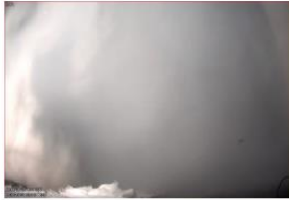
Novec 1230 discharge [TR + 00:00:58]
