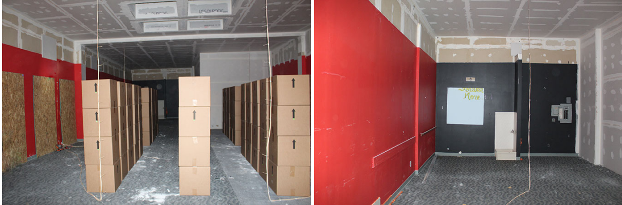
Figure 2.17: Interior images of unit 1067, looking toward side C from the front entry door (left), and toward side C from two-thirds of the way into the space (right).
