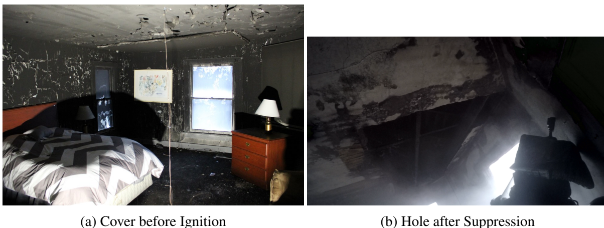
Figure 3.152: Interior photographs of the failed ceiling prior to ignition (see Figure 3.152a) and after suppression (see Figure 3.152b) for Experiment 13.
