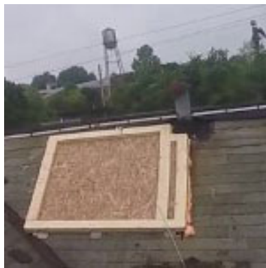
(a) Roof Vent
