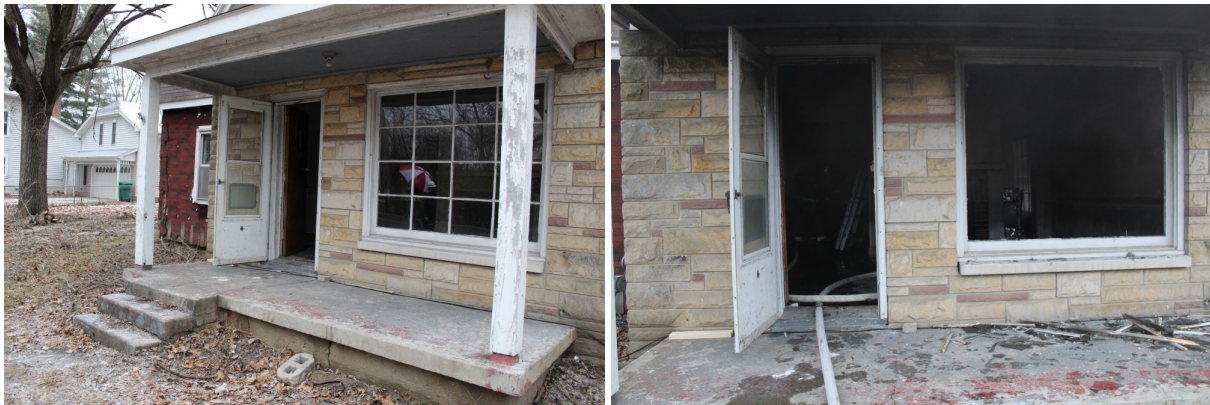
(a) Before Ventilation
