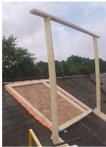
(a) Roof Vent
