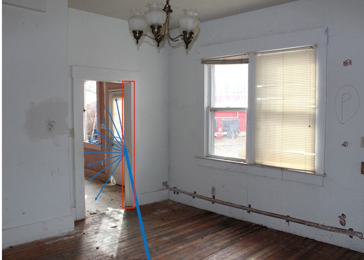
Figure 5.19: Interior view along the entry path looking toward the fire compartment (a kitchen). Note: The doorway king stud highlighted in red.
