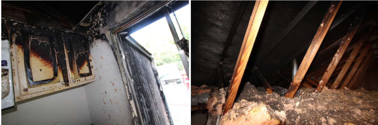
(a) Extension Damage to Second-floor Kitchen
