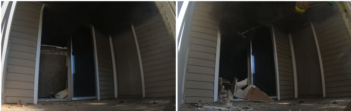
(a) Fallen Drywall Blocking the Sliding Glass Door
