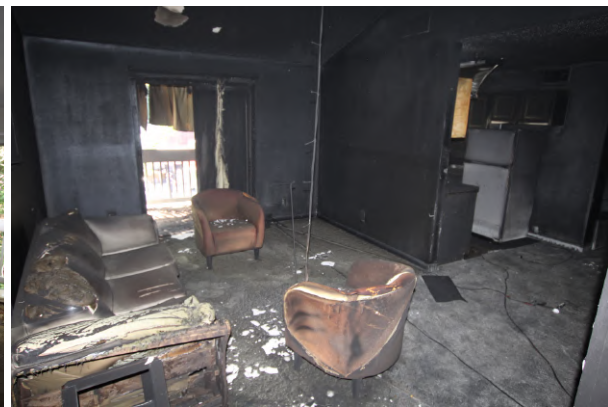
(b) Apartment F (Non-Isolated) Post Fire
