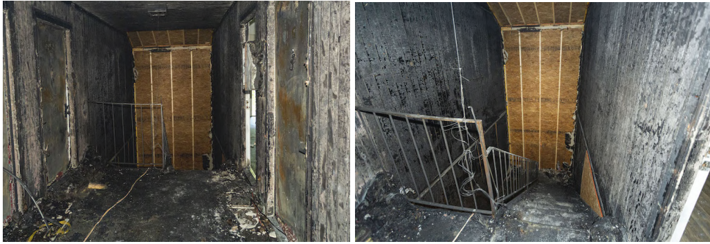
(a) Warped Railing
