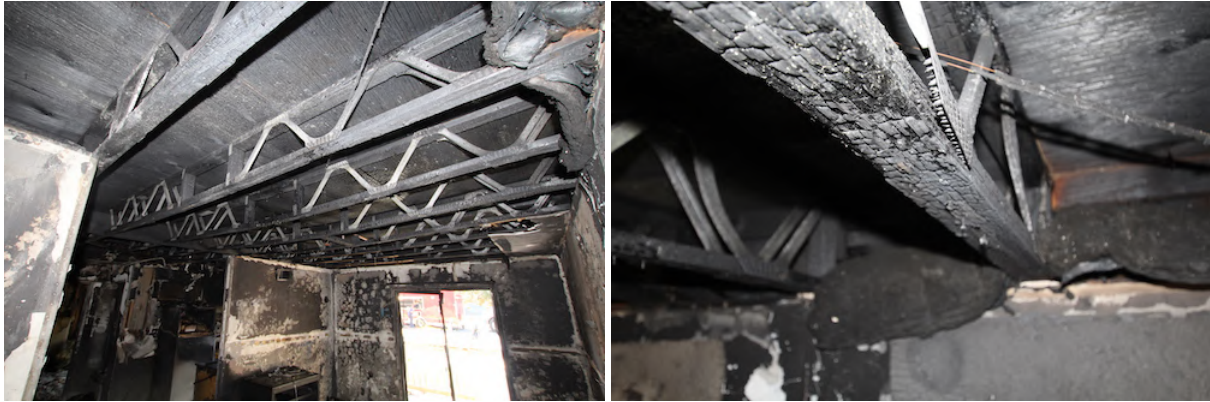
(a) Sagging Ceiling
