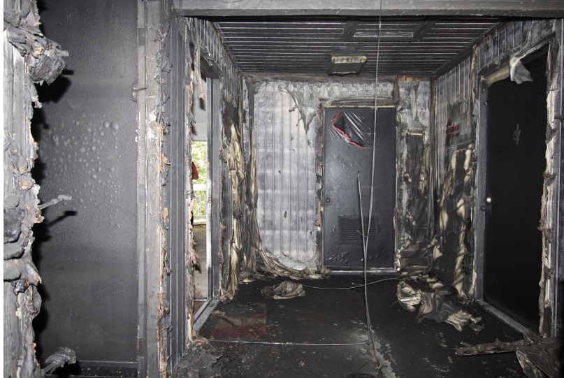
Figure 5.16: Post fire conditions as seen from the second-floor landing in Experiment 5. Note the extreme damage to the area with a limited view into Apartment H, which was isolated early into the experiment, maintaining survivable space.
